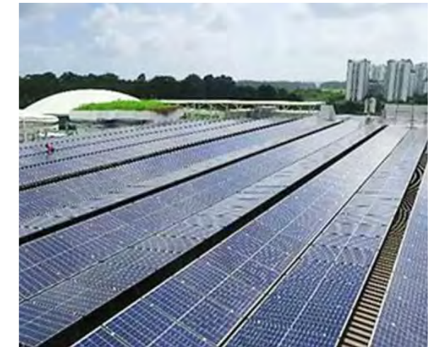
Project Location: Singapore Capacity: 221Wp Completion Year: 2017 Type: Metal roof Mounted
