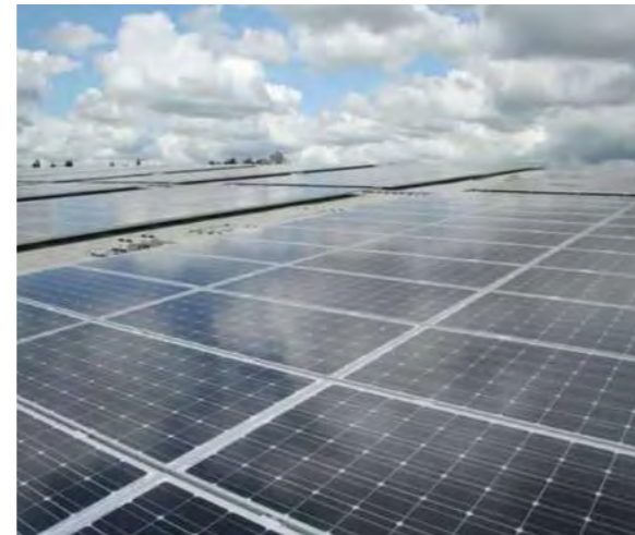
Project Location: Klang, Malaysia Capacity: 426kWp Completion Year: 2016 Type: Metal roof Mounted
