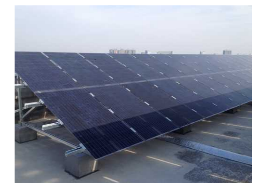
Project Location: Cebu, Philippines Capacity: 2.5MWp Completion Year: 2017 Type: RC Roof Mounted
