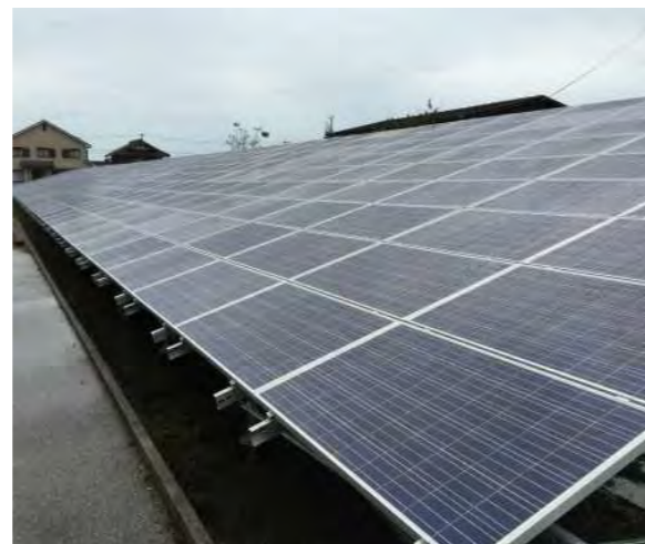
Project Location: Shiga-ken, Japan Capacity: 2MWp Completion Year: 2015 Type: Ground Mounted
