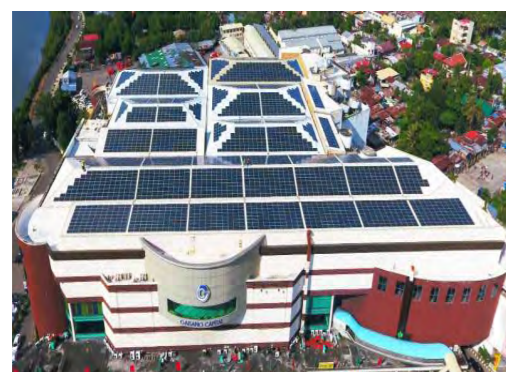
Project Location: Iloilo, Philippines Capacity: 1.9MWp Completion Year: 2016 Type: Metal roof Mounted
