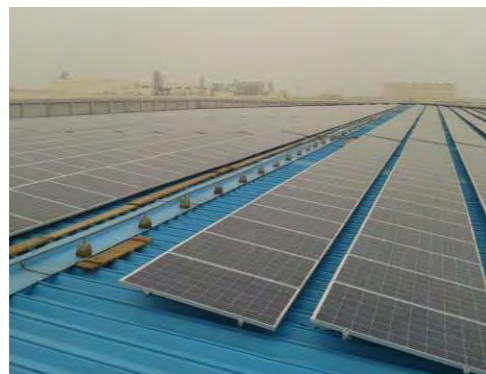
Project Location: Singapore Capacity: 1.6MWp Completion Year: 2017 Type: Metal roof Mounted
