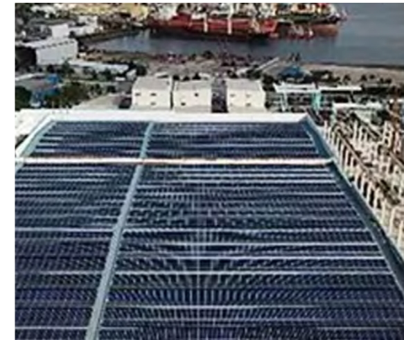
Project Location: Tuas, Singapore Capacity: 1MWp Completion Year: 2017 Type: Metal roof Mounted
