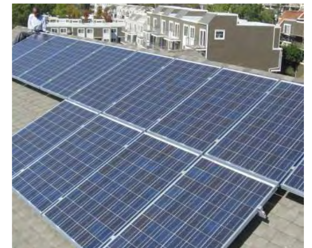
Project Location: USA Capacity: 2.5MWp Completion Year: 2015 Type: RC roof Mounted
