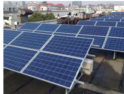
Project Location: Shanghai, China Capacity: 4.3MWp Completion Year: 2016 Type: Concrete Roof Mounted
