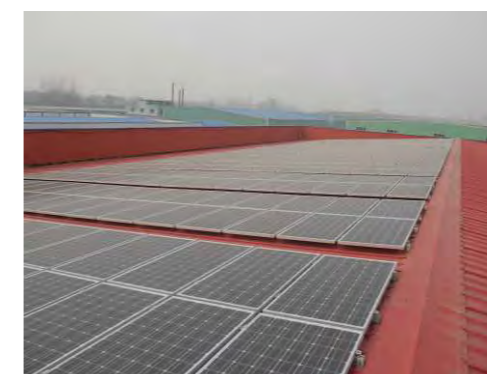
Project Location: Iloilo, Philippines Capacity: 1.9MWp Completion Year: 2016 Type: Metal roof Mounted
