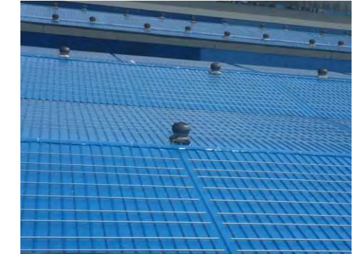
Project Location: Singapore Capacity: 221Wp Completion Year: 2017 Type: Metal roof Mounted
