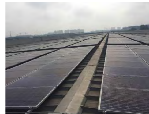
Project Location: Shiga-ken, Japan Capacity: 2MWp Completion Year: 2015 Type: Metal Roof Mounted
